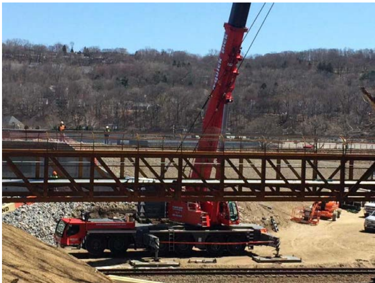
Figure 16 Ansonia Riverwalk Park, pedestrian bridge construction April 2018, Photo by Michael P. Mayko CTPOST
