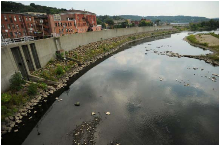
Figure 5 Ansonia, CT 2015, Flood Wall, Photo by Brian A. Pounds - Hearst CT Media
